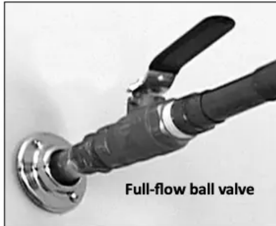
Figure 17 - Fully open the cold water supply valve.
