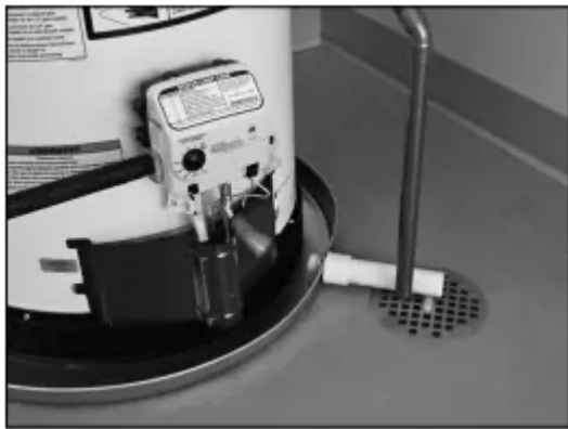
Figure 23 - Metal drain pan piped to drain.
