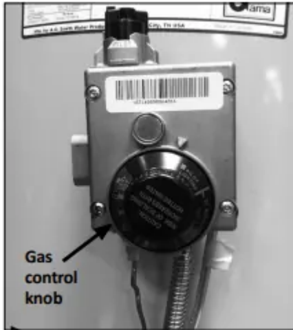
Figure 17 - Turn gas control/temperature knob OFF.
