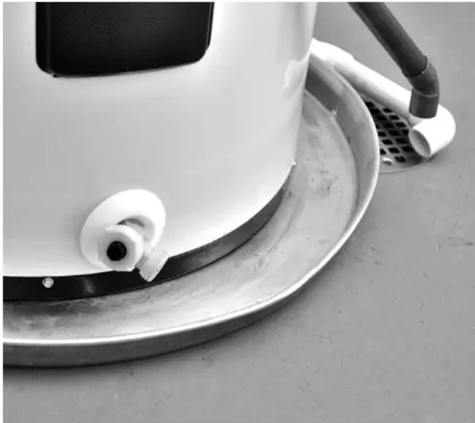
Figure 6 - A suitable drain pan piped to an adequate drain can help protect flooring from leaks and drips.
