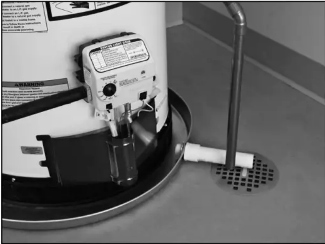
Figure 23 - Metal drain pan piped to drain.
