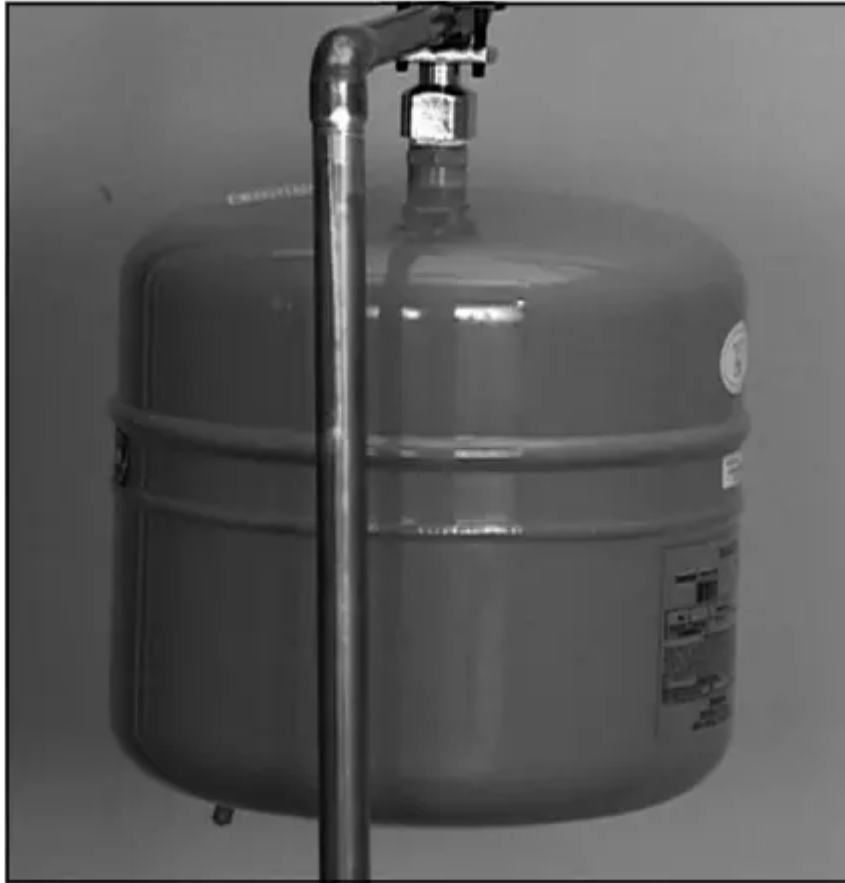
Figure 5 - A Thermal Expansion Tank helps protect the home's plumbing system from pressure spikes.
