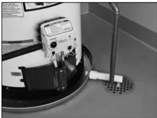
Figure 23 - Metal drain pan piped to drain.
