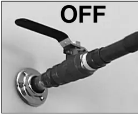
Figure 19 - Cold water supply in off position.
