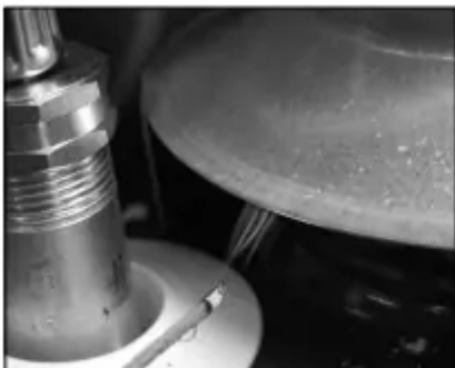
Figure 35 - Test the air supply and vent to make sure the water heater has adequate air and is venting properly.
