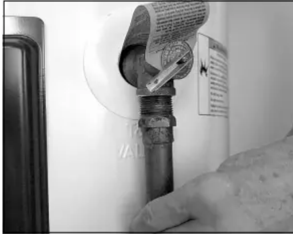
Figure 12 - The T&P Relief Valve discharge pipe must be installed properly and piped to an adequate drain.
