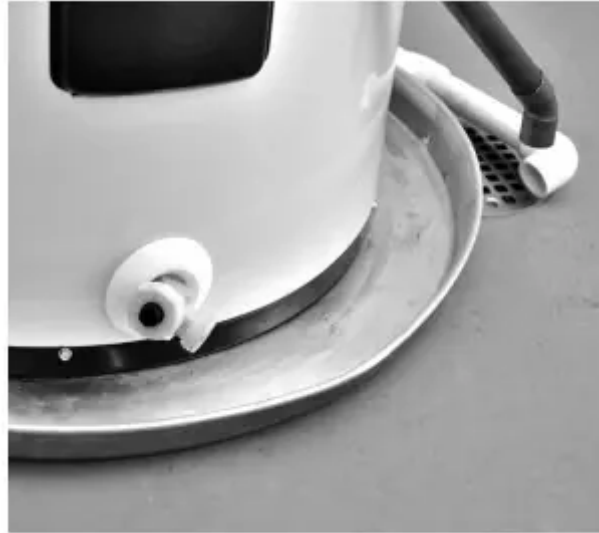
Figure 6 - A suitable drain pan piped to an adequate drain can help protect flooring from leaks and drips.
