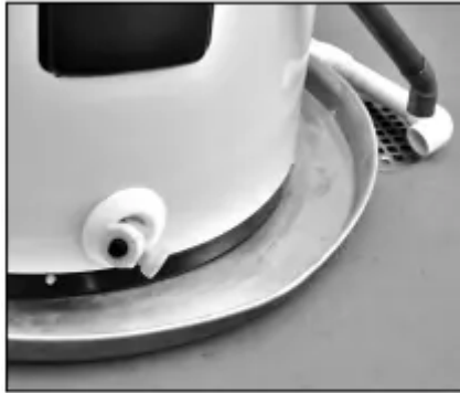
Figure 6 - A suitable drain pan piped to an adequate drain can help protect flooring from leaks and drips.
