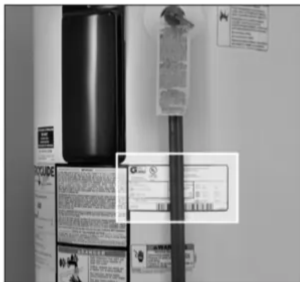
Figure 18 - The water heater's electrical requirements can be determined from the data plate.
