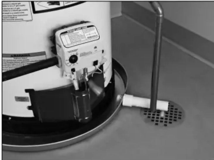
Figure 23 - Metal drain pan piped to drain.
