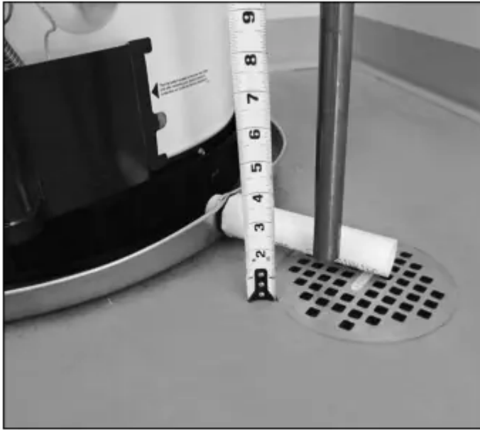
Figure 26 - Temperature and Pressure Relief Valve Pipe
