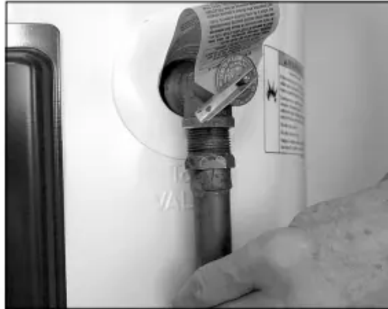
Figure 12 - The T&P Relief Valve discharge pipe must be installed properly and piped to an adequate drain.
