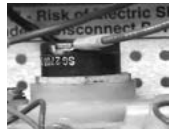
Figure 11: Installed heating element
