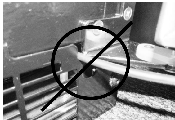
INCORRECT WIRE POSITION.
