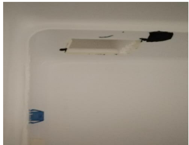
Freezer → air supply outlet of fridge
