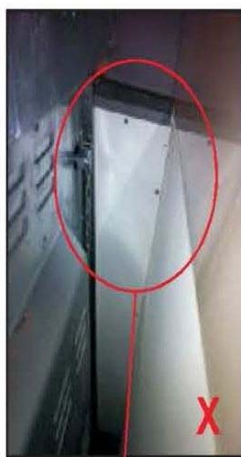
Left Side of oven, chain not attached
