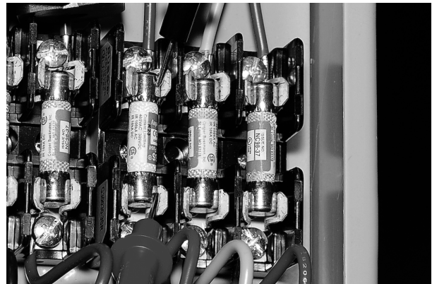
Figure 11. Fuse Test - Volt Meter Method
