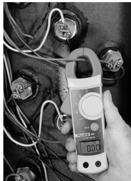
Figure 18. Heating Element Amperage Test
