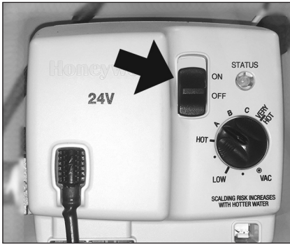
Figure 37 - Turn gas control/temperature knob OFF.
