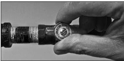
Figure 32 - Gas valve in "on" position
