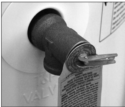
Figure 25 - Temperature and Pressure Relief Valve
