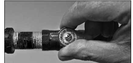
Figure 50 - Gas valve in “on” position.
