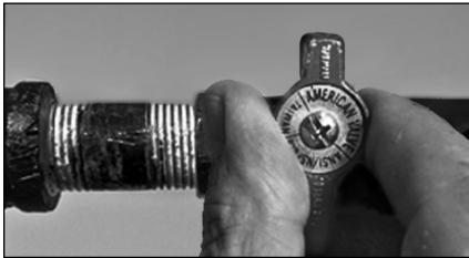
Figure 46 - Gas valve in “off” position.
