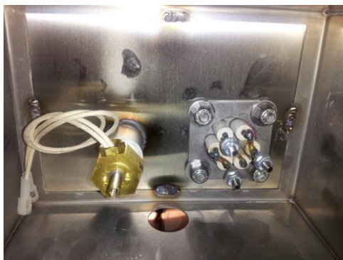
Showing thermostat and sustainer heater terminals*
