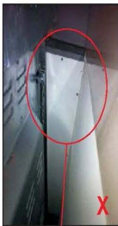
Left Side of oven, chain not attached
