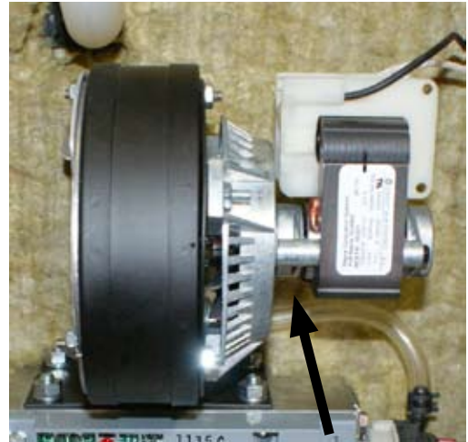
Fan Pressure Switch Hose
