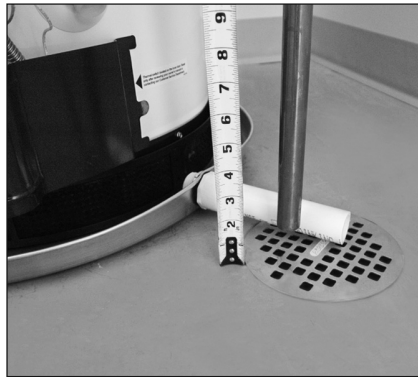
Figure 26 - Temperature and Pressure Relief Valve Pipe
