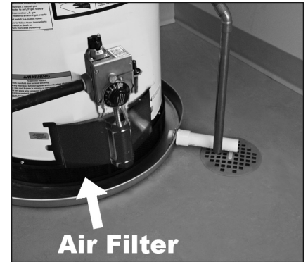
Figure 24 - Filter attached to water heater.
