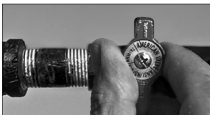
Figure 46 - Gas valve in “off” position.
