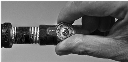
Figure 32 - Gas valve in "on" position
