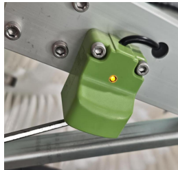
左侧接近开关（常亮） Left-side proximity switch (normally illuminated)
