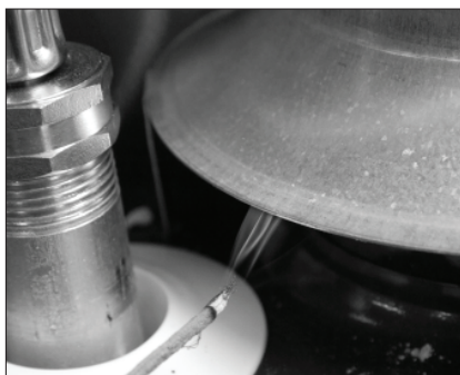
Figure 32: Test the air supply and vent to make sure the water heater has adequate air and is venting properly.
