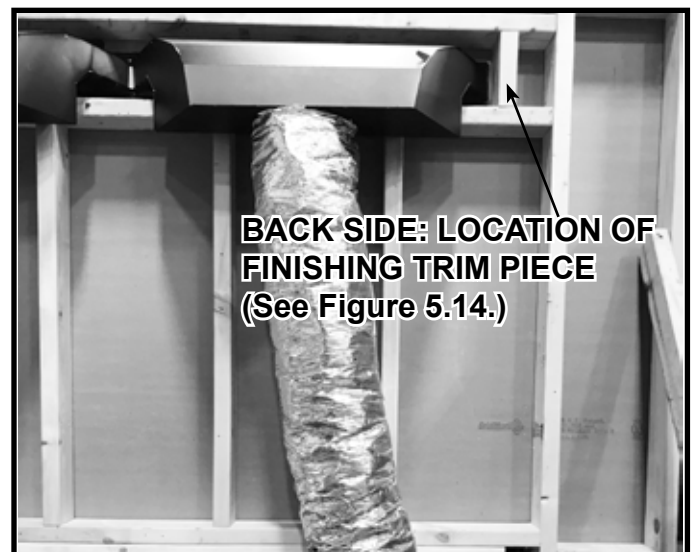
Figure 5.29 Flex Vent Installed with No Kinks
