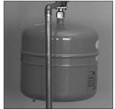
Figure 20 - The Thermal Expansion Tank should be pressurized with air, to match the home's incoming water pressure.
