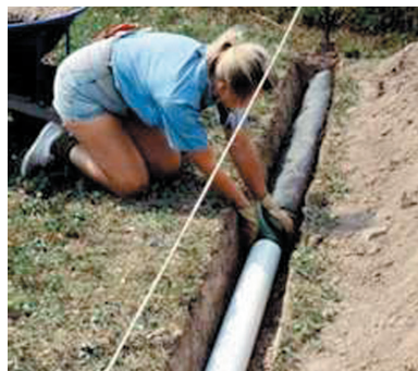
Figure 33: Underground Refrigerant Piping.
