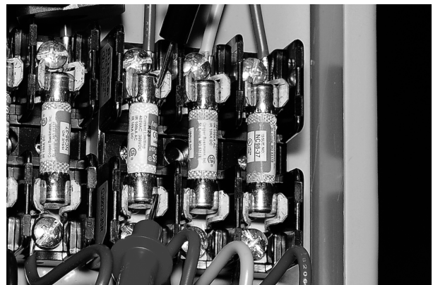
Figure 11. Fuse Test - Volt Meter Method
