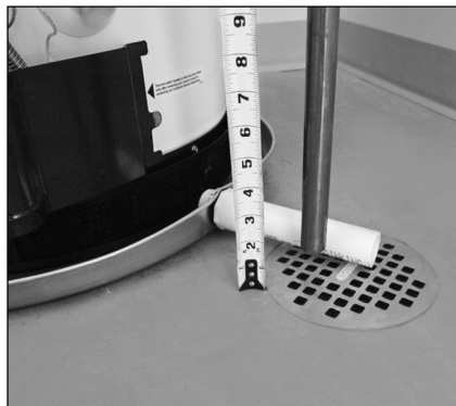
Figure 26 - Temperature and Pressure Relief Valve Pipe
