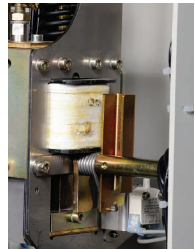
Interlock blocked (cover removed for photo)
