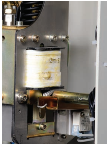
Interlock not blocked (cover removed for photo)
