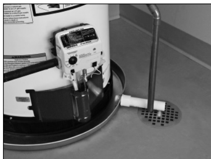
Figure 23 - Metal drain pan piped to drain.
