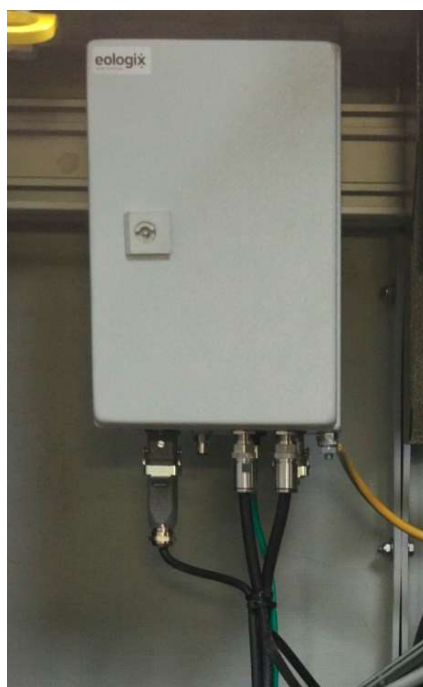
Figure 13 Example of a cabling (previous version)
