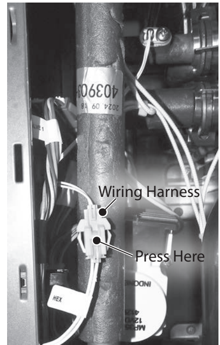
Figure 76 - Wiring harness location
