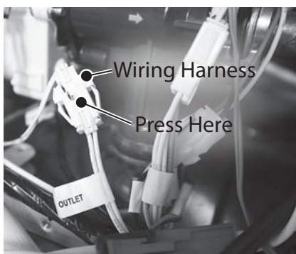
Figure 73 - Wiring harness location
