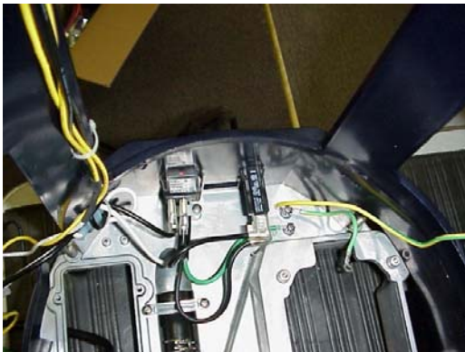
Figure 19. Power switch and circuit breaker.
