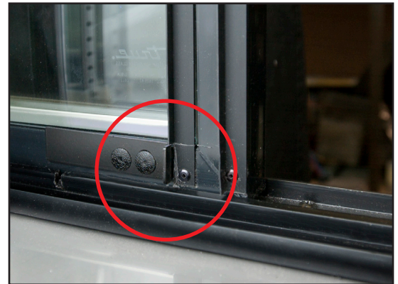
Fig. 2. Door latch is in the closed position (disengaged from notch).
