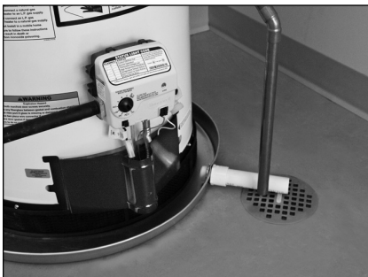
Figure 23 - Metal drain pan piped to drain.
