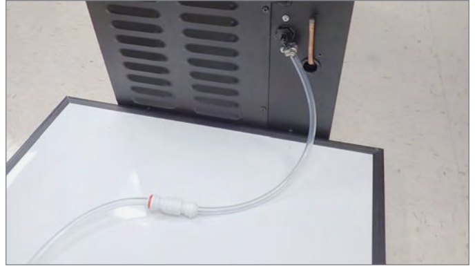
FIG. 6. Installed check valve.
