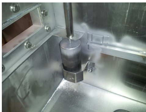
Wash tank float and tank overflow
