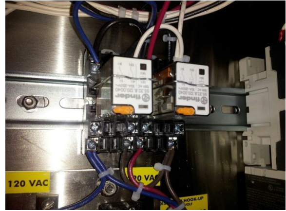
Conveyor motor control relays
