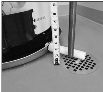
Figure 26 - Temperature and Pressure Relief Valve Pipe
