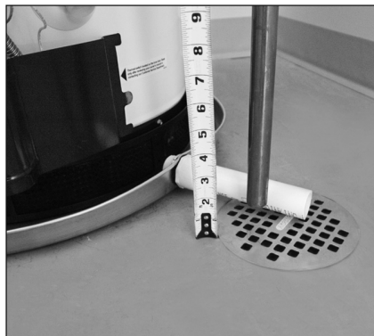
Figure 26 - Temperature and Pressure Relief Valve Pipe
