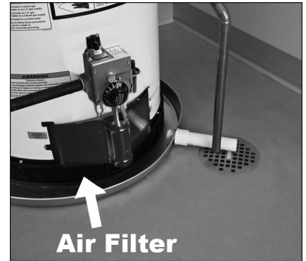
Figure 24 - Filter attached to water heater.
