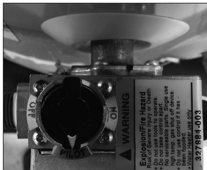
Figure 34 - Gas control/valve top view.
