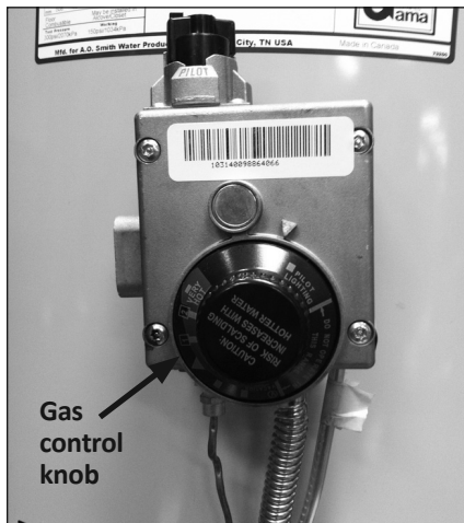
Figure 17 - Turn gas control/temperature knob OFF.
