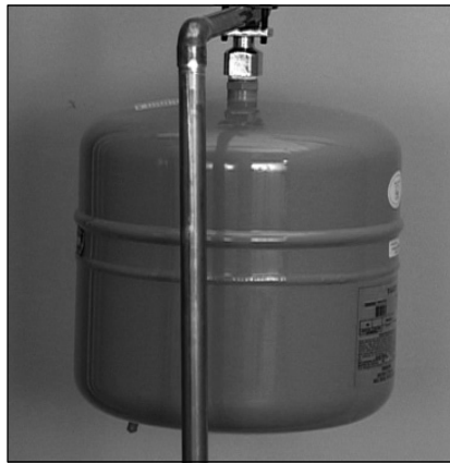
Figure 29 - The Thermal Expansion Tank should be pressurized with air, using a hand pump, to match the home's incoming water pressure.
