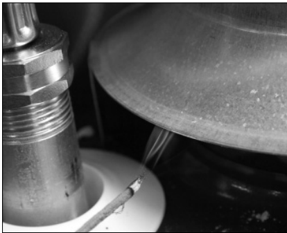
Figure 36 - Test the air supply and vent to make sure the water heater has adequate air and is venting properly.
