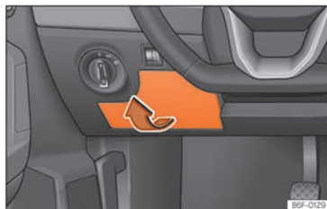
Fig. 159 On the dashboard on the driver side: lid of the fuse box.
