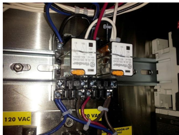
Conveyor motor control relays
