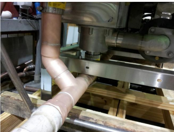
Showing 2" drain manifold exiting sump & scrap box
