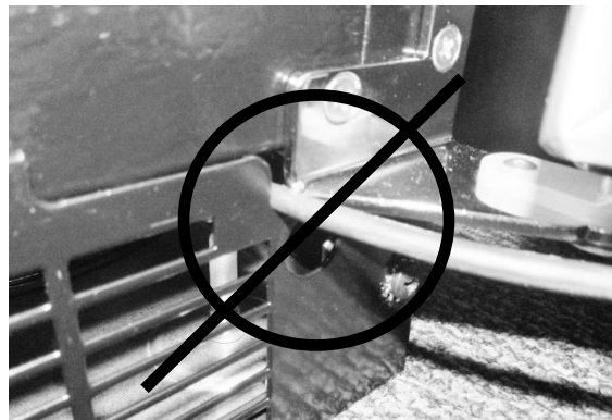
INCORRECT WIRE POSITION.
