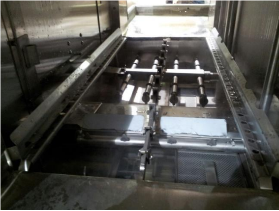
Travel through conveyor tray rails, center pull bar w/dogs
