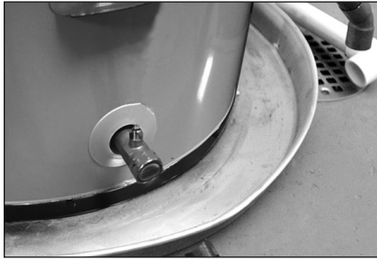
Figure 6 - A suitable drain pan piped to an adequate drain can help protect flooring from leaks and drips.
