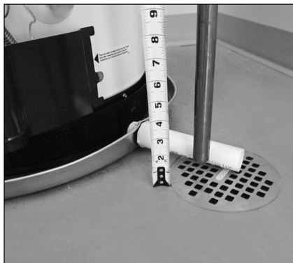
Figure 26 - Temperature and Pressure Relief Valve Pipe
