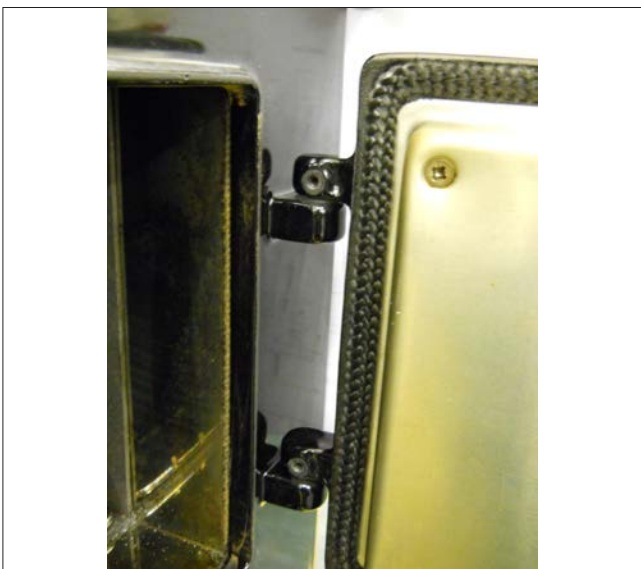
Fig 15 DOOR HINGES LOCATED
