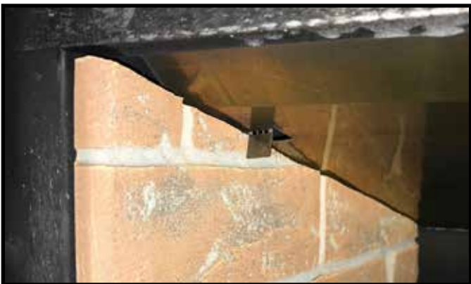
Figure 6 Left Refractory Handbend Tab
